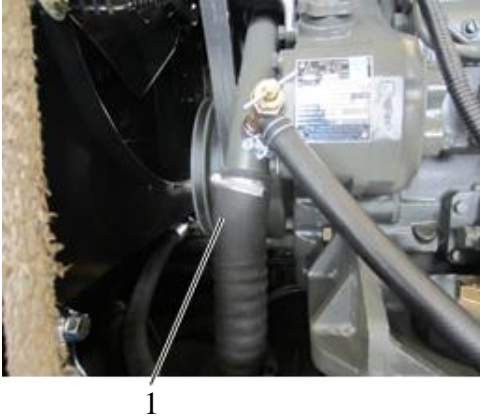
Fig. 2-28 1 Return pipe of engine
