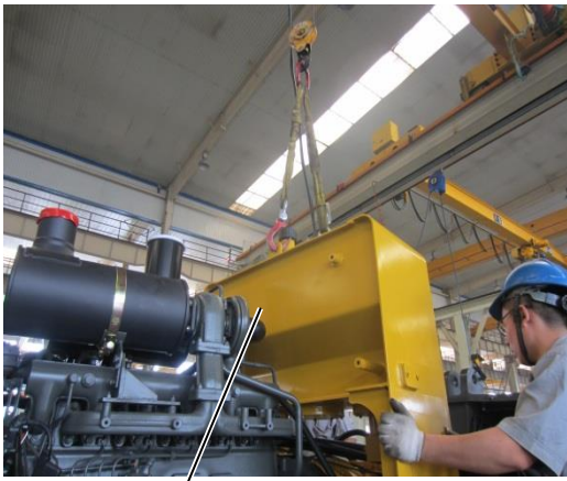
1 Fig. 2-14 1 Hydraulic oil tank
